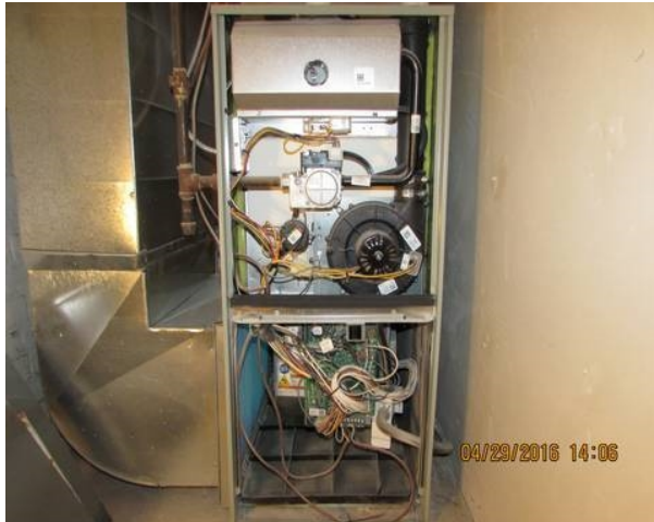
High efficiency furnace
