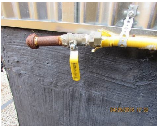
External Gas shut off
