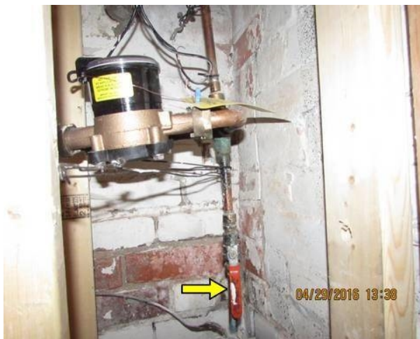
Water meter and main shut off
